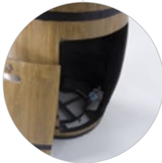
Concealed Propane Tank
